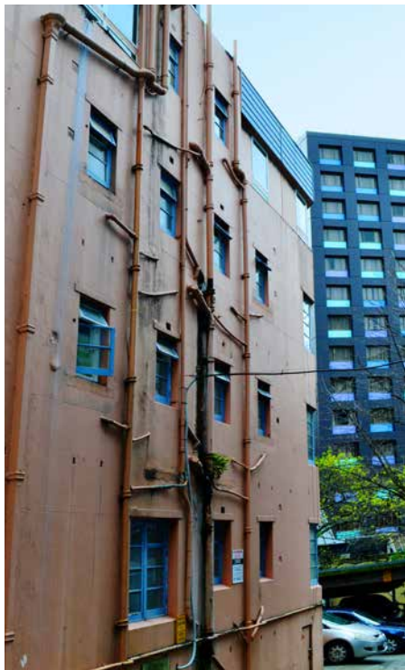
Plumbing issues prior to the refurbishment
